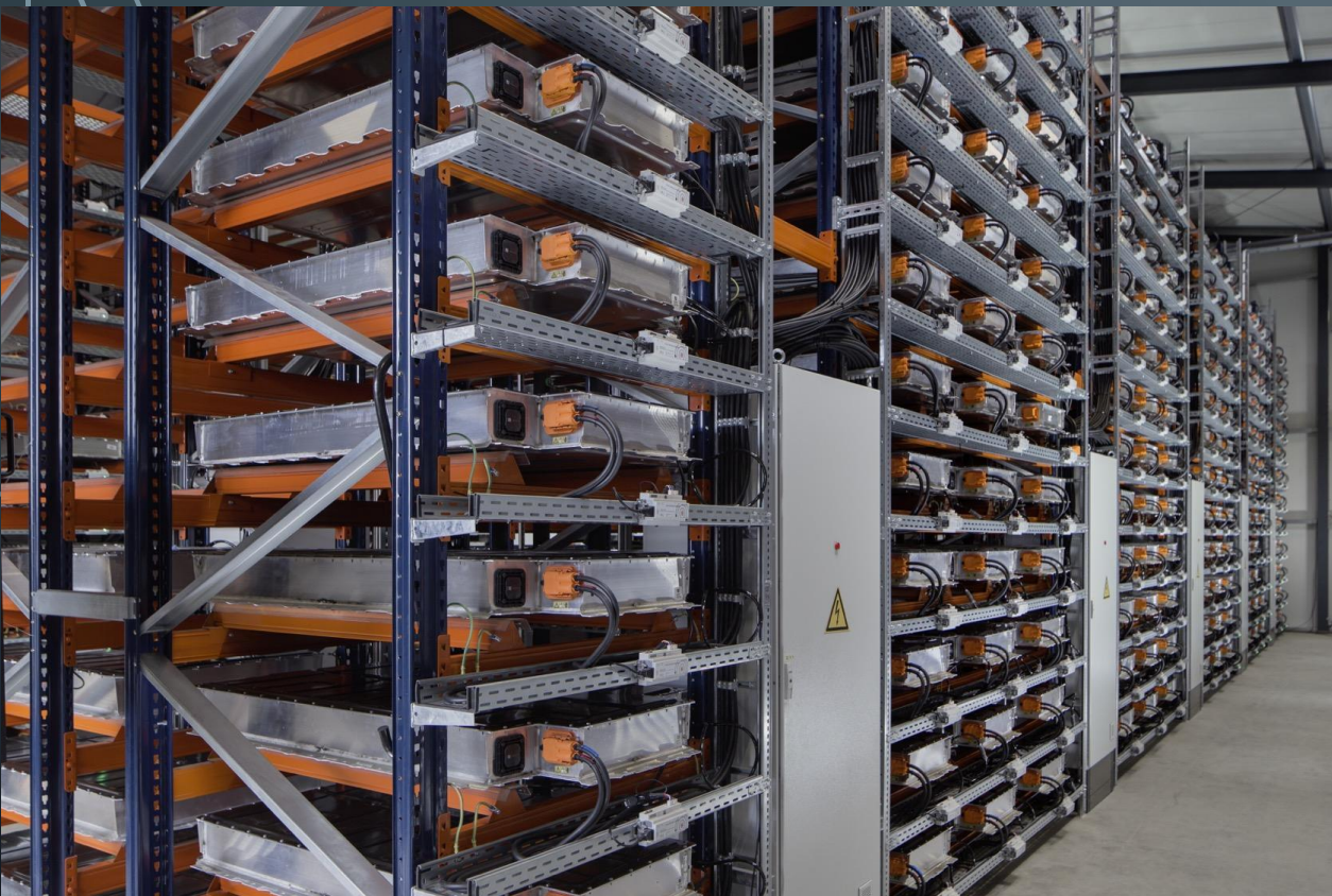
Armazenamento de energia, BMW Plant Leipzig, Germany
